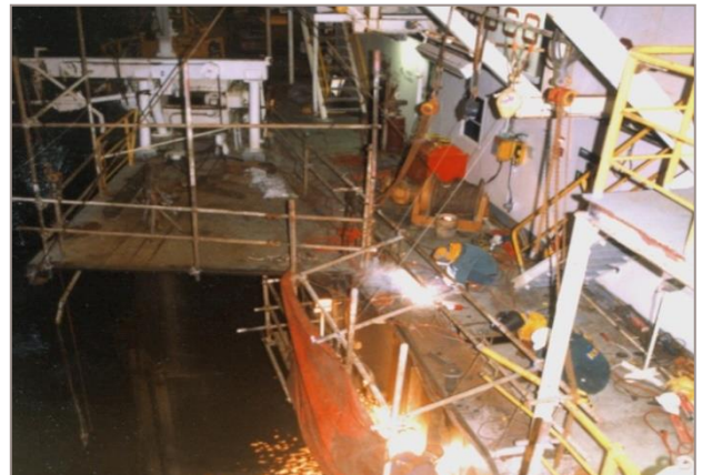
After the damaged platform was removed repair work was done on the man girder
