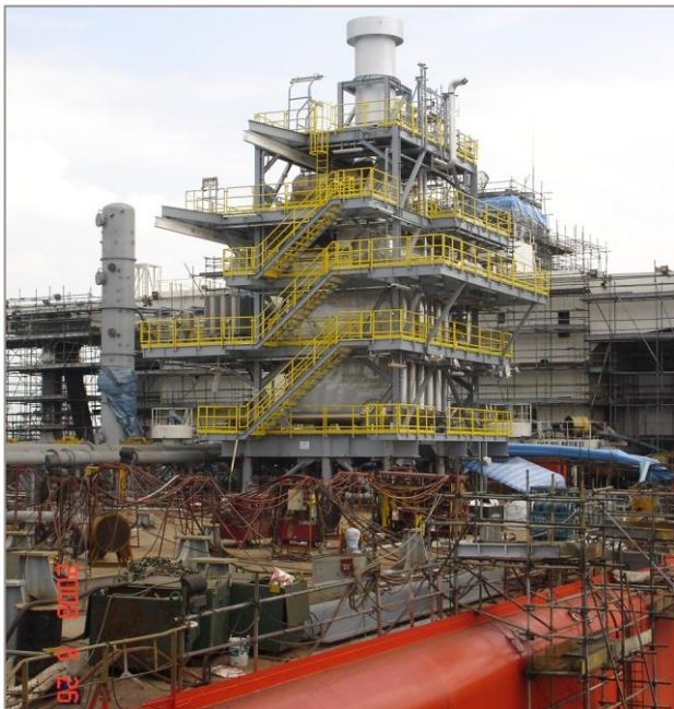
Aalborg boiler module installed on Azurite FDPSO
