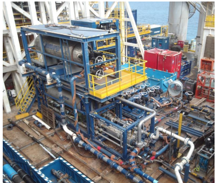
Steam exchanger stacked onto separator
