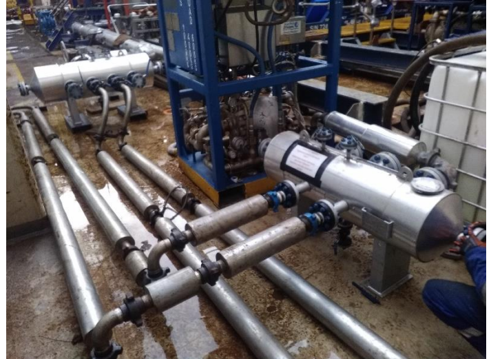
Steam manifolds and insulated pipework for steam exchanger
