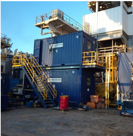
Sampling lab cabin stacked onto data acquisition cabin
