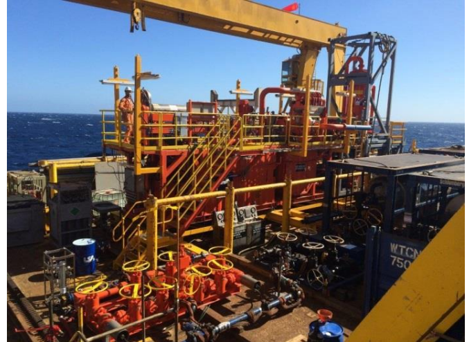
The PFMS installed on the Atwood Eagle
