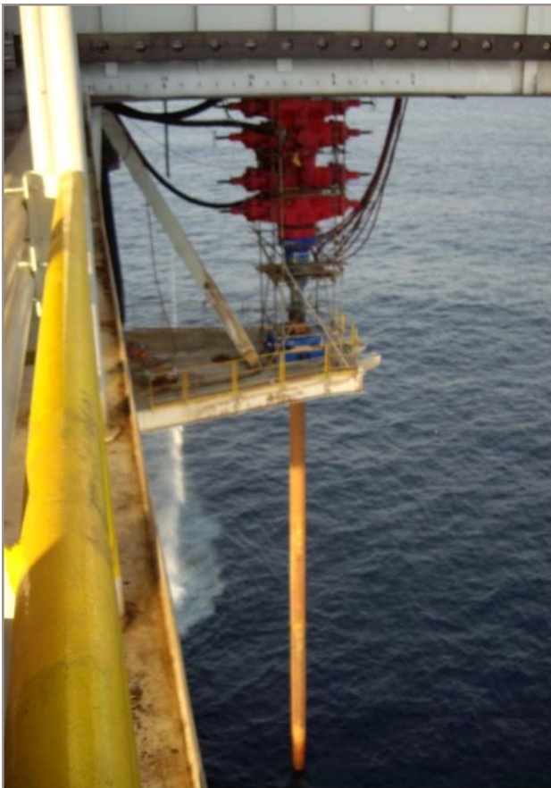
Typical conductor installation
