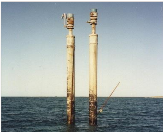
A pair of "Minnowpod" conductors, completed and suspended, awaiting installation of topsides
