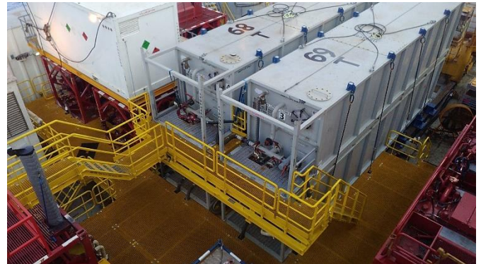
Gravel Pack Spread Support and Access Structure as installed
