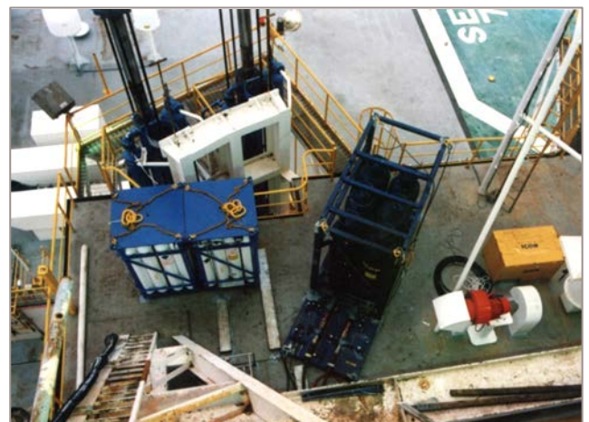
View on the air accumulator modules and valve skid
