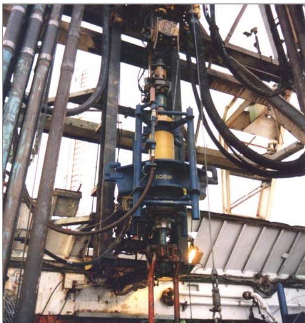
View of the compensator cylinder installed on the Sedco 703 MODU
