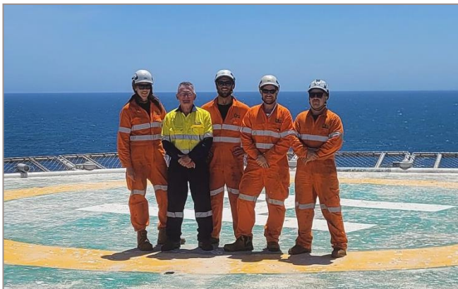
The ICON team which hand carried and installed replacement grating and structural steel on the legacy CHA platform.
