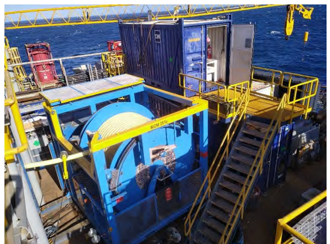
Intervention Workover Control System (IWOCSS) spread installed by ICON.
