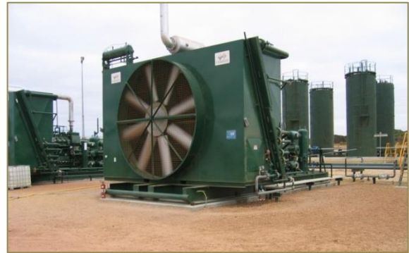
Two Waukesha Gas Engine-Driven (1215 hp) Ariel Compressors used for Gas Lift at ARC's Hovea Facility.
