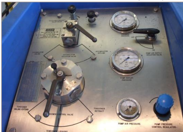
Operators' Control Panel
